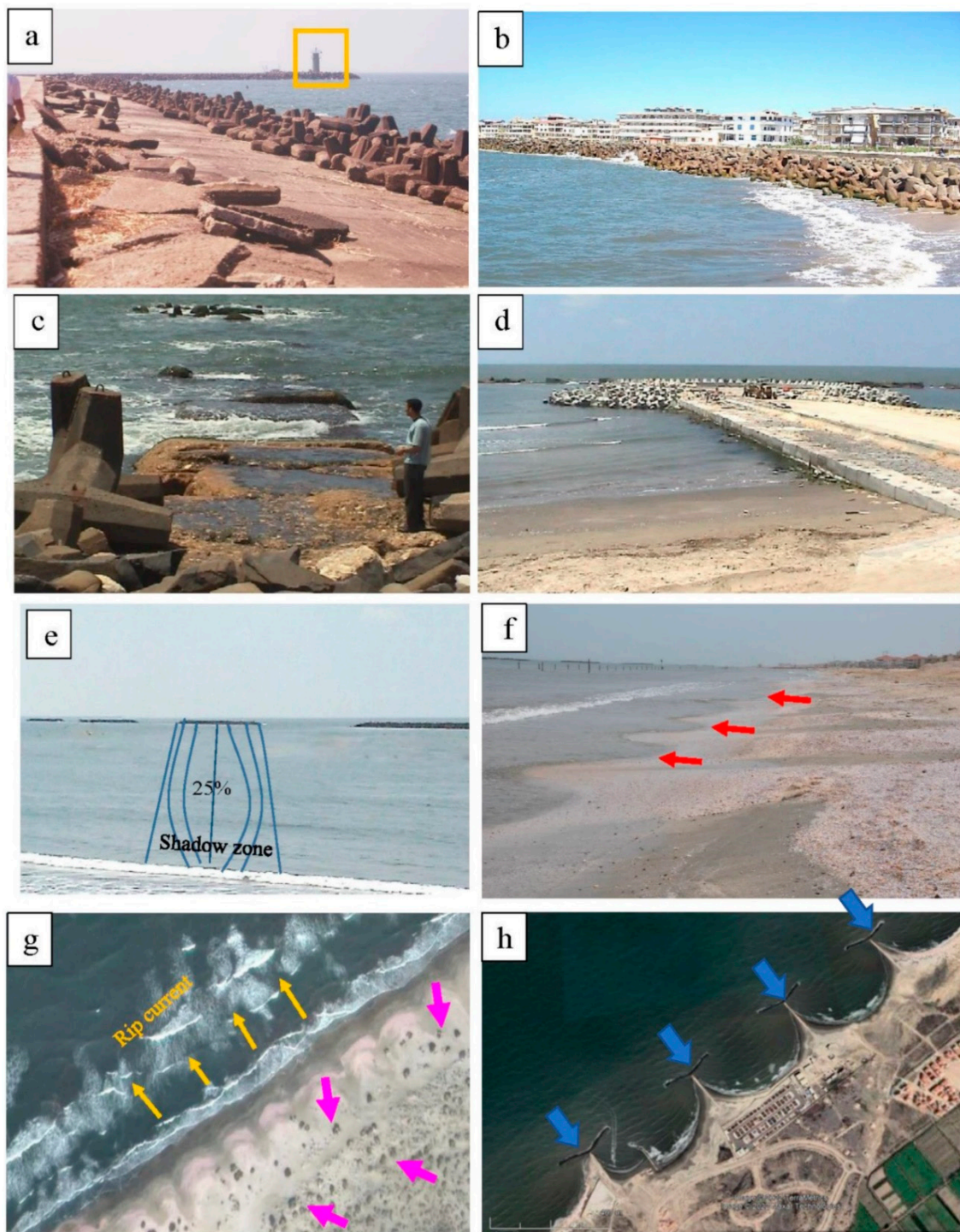
Figure 5. The coast west of the promontory at Ras El-Bar showing the concrete seawall. (a) The yellow rectangle refers to the lighthouse; the modified 1200 m seawall extends westward of the Damietta Nile branch. (b) One of the three 120 m long concrete groins that were constructed to the west of the seawall at “b” and (c) later renewed. (d) The successful detached breakwaters that create shadow zones of 25% of the waves’ energy. (e) Eastward evidence of erosion including shell accumulation, cusped beach “red arrows” (f) at the coast east of the harbor eastern jetty (see Figure 1c yellow area), with developed rip currents (yellow arrows) (g) and waves rolled mud balls along the eroded coast (pink arrows) (g), [4]. The new Y groins east of the harbor jetty (blue arrows) (h) with accretion along the groins and erosion along the spaces in between.
