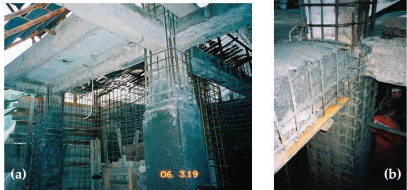
Figure 1. (a) RC jacket of columns employing shotcrete (gunite). (b) RC jacket of column and beam at the region of their joints employing shotcrete (gunite) [13].
