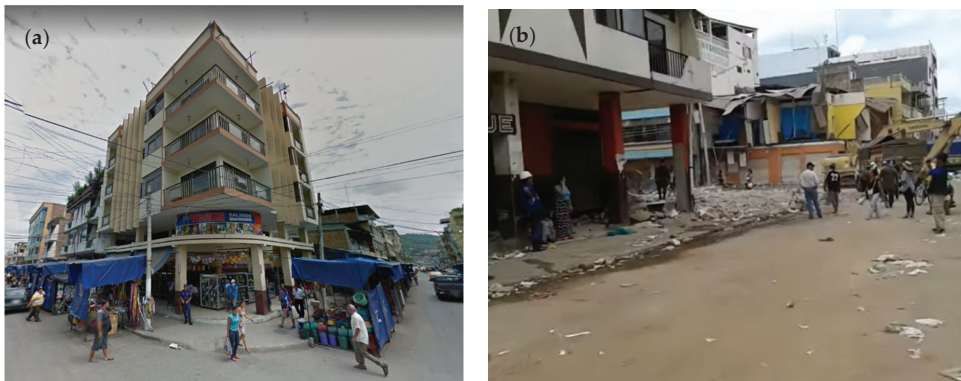
Figure 2. Marinero building located on Chile Street in Portoviejo, (a) before the earthquake and (b) after the earthquake.
