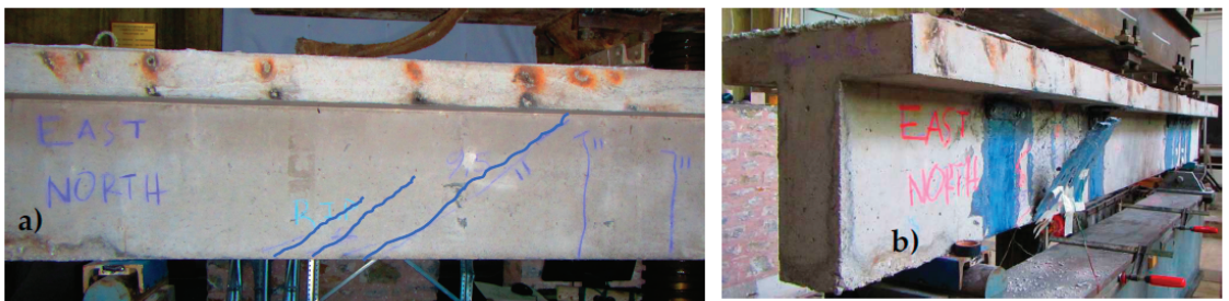
Figure 17. Comparison of failure modes between the prototype RC Virgin T-beam and this T-beam having been retrofitted with the 1st strengthening scheme. (a) Diagonal shear cracks at the East part of the Virgin T-beam. (b) The debonding of two open hoop CFRP strips without anchoring at the East part of this T-beam retrofitted with the 1st strengthening scheme.
