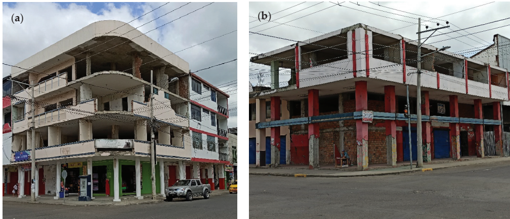
Figure 1. Current status of damaged buildings located on the corners of Chile Street, Portoviejo (a) building in use and (b) building closed.
