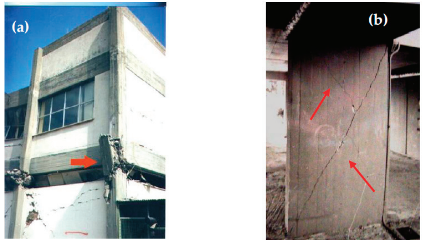
Figure 3. (a) Shear failure of an RC short column at the ground floor of a two-story RC building. Aigio, Greece 1995 earthquake sequence. (b) Detail of shear damage of a shear wall at the ground floor of a four-story RC building. Pyrgos, Greece 1993 earthquake sequence [1].
