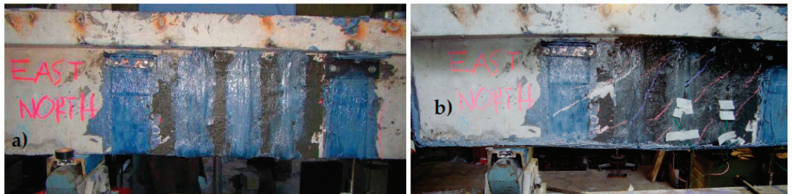
Figure 19. (a) The 2nd strengthening scheme (East part). (b) Diagonal shear cracks at the East part of the prototype RC T-beam, which were checked by the applied CFRP anchor poles.
