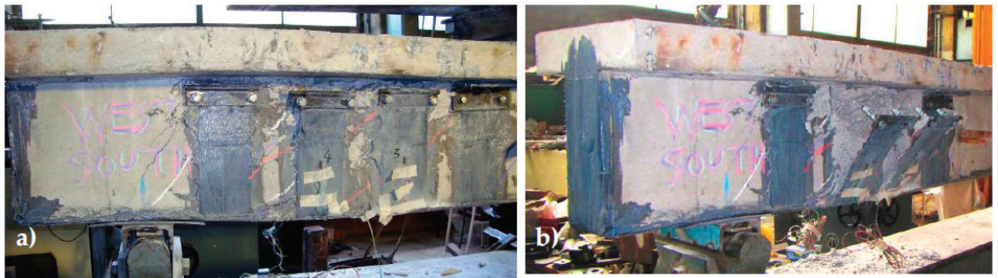
Figure 23. (a) The 3rd strengthening scheme (West part). (b) The widening of the shear diagonal cracks and the partial crushing of the concrete volume in the anchoring region reduced considerably the effectiveness of this anchoring scheme.
