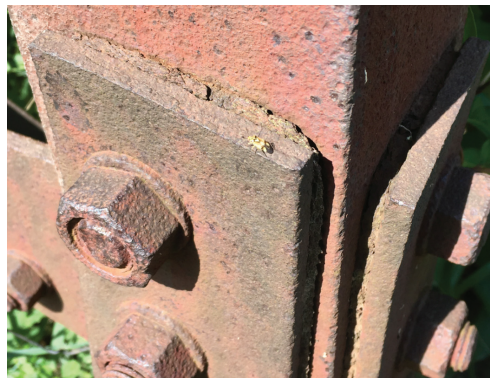
Figure 16. Crevice corrosion at the bolted joint of leg members (Locality 5).
