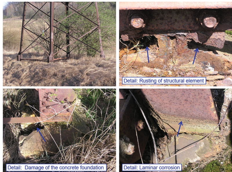
Figure 24. Selected examples of corrosion damage in the anchorage area of transmission towers.
