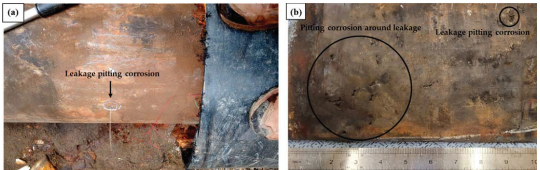
Figure 2. Photographs of the failed pipe: (a) water leakage resulting from pitting in the failed pipe, (b) external surface of the failed pipe around the leakage area.
