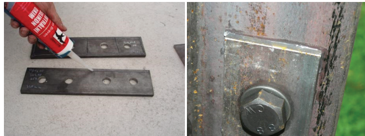
Figure 8. Application of silicone sealant ((left) application of sealant to the splices; (right) sealant smoothed around the perimeter of the splice).
