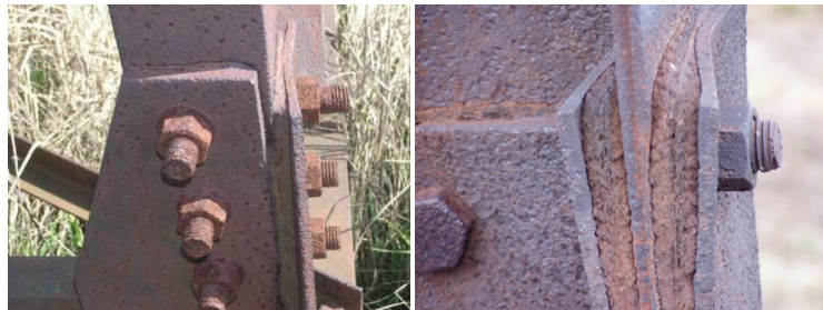
Figure 1. Crevice corrosion in the bolted joint of the leg member.
