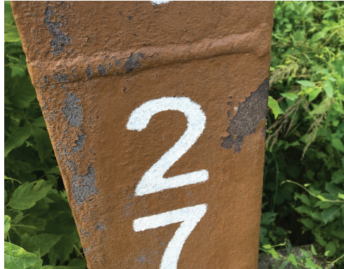
Figure 17. Failure of a paint system applied to a poorly prepared surface (the original protective layer of corrosion products remains under the peeling paint).
