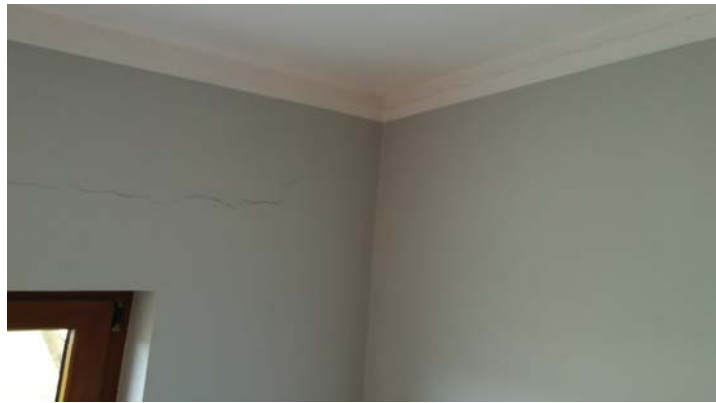
Figure 20. An example of a crack was created as a result of uneven settlement of the building (at the window and under the ceiling).
