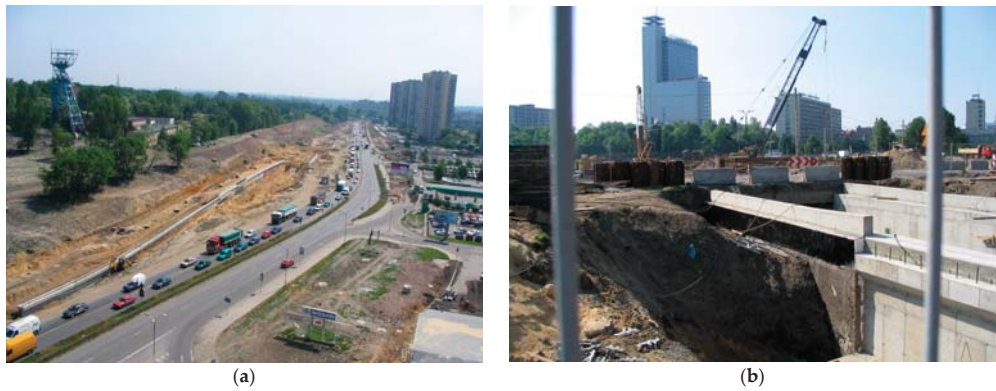
Figure 7. Execution of works as part of the construction of the tunnel under the Roundabout in Katowice: (a) beginning of the tunnel; (b) construction of diaphragm walls.
