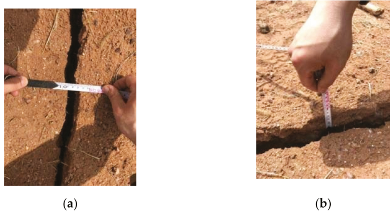
Figure 10. Surface crack drop and width measurement:(a) Measurement of ground crack tension; (b) Ground crack step drop measurement.
