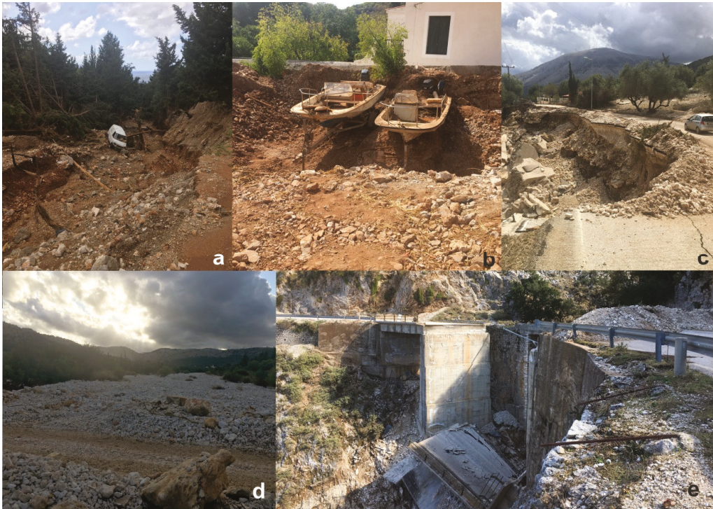
Figure 11. Characteristic damages in Cephalonia Island following Medicanne Ianos: (a) Riverbank erosion, (b) debris flow within a rural community, (c) road embankment failure, (d) extensive debris flow, and (e) bridge collapse.
