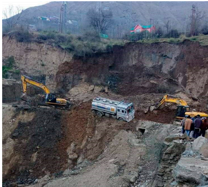
Figure 2. Prominent landslide site at Ramban along the NH 44.
