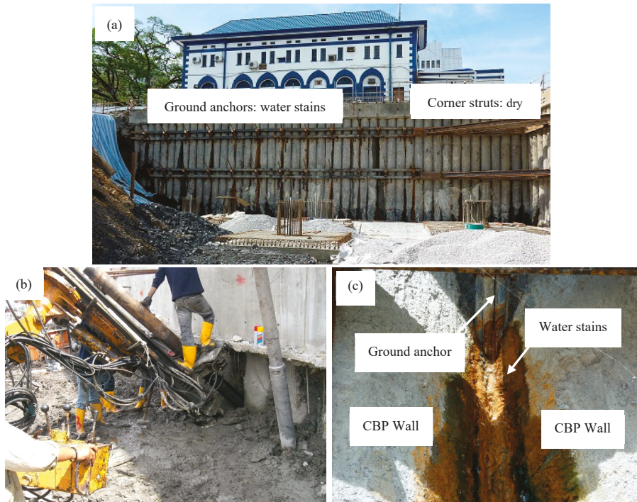
Figure 7. (a) Groundwater leakage from where ground anchors were installed; (b) drilling of ground anchor in between bored piles; and (c) close-up of the water leakage from the ground anchor.
