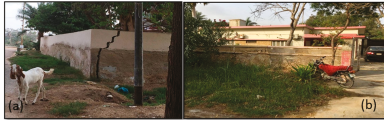
Figure 10. Signs of ground displacements in the study area. (a) Cracks in the building walls due to differential ground displacement; (b) elevation of a residential house in the University of Karachi's Professors colony has dropped to ~2 m below its base-level due to soil liquefaction caused by seawater intrusion. During the field visit, signs of soil salinity were observed in different parts of the University of Karachi.
