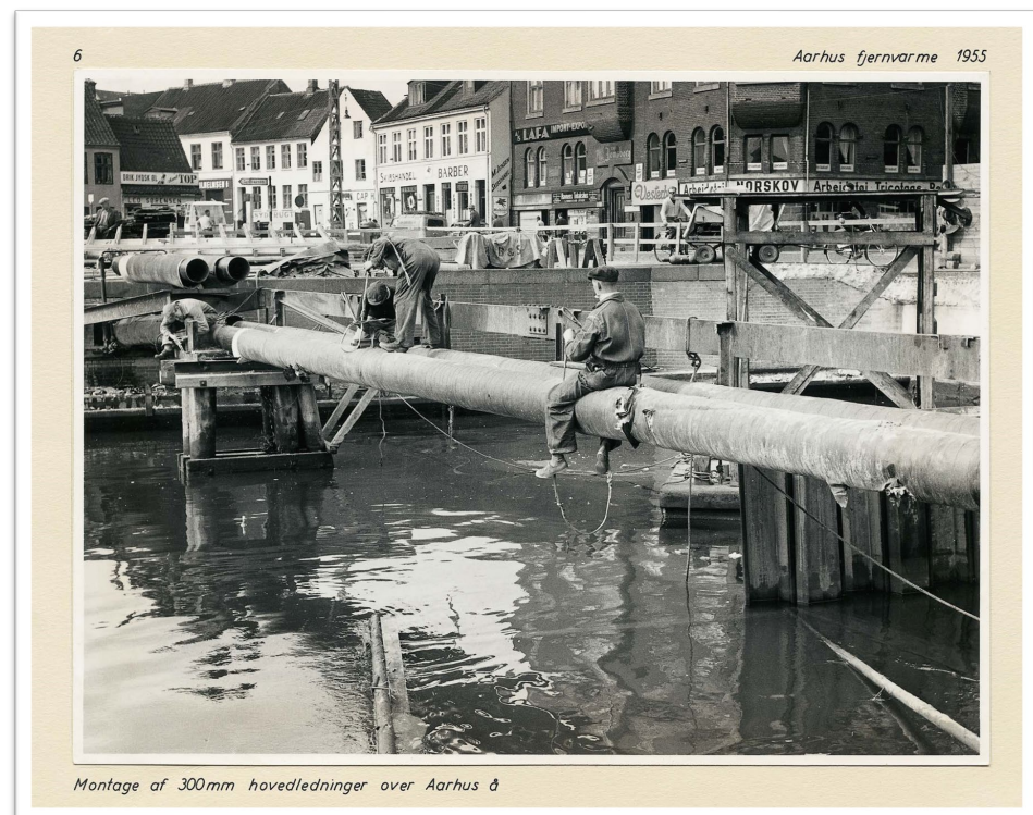
Figure 4. Deployment of 300 mm main pipes across the water in Aarhus, 1955. Source: Affaldvarme Aarhus; this was printed with permission.
