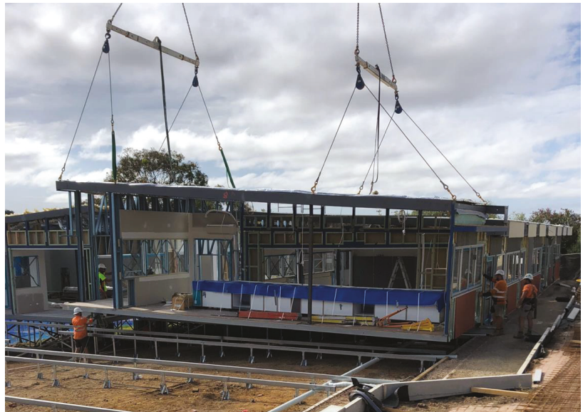
Figure 18. A partially finished modular unit being installed on top of a prefab foundation (driven in piles with a base plate and steel bearers on top).
