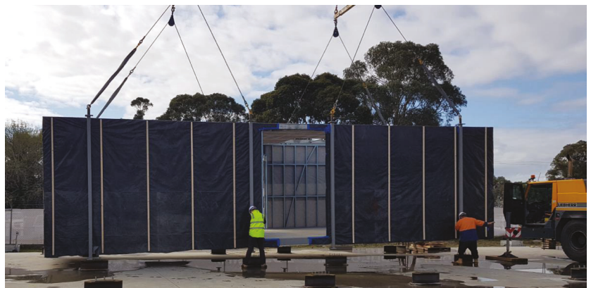
Figure 7. A partly finished structural module being lifted into place using a top-lift method where the lifting mechanism is properly connected to full-length structural columns.
