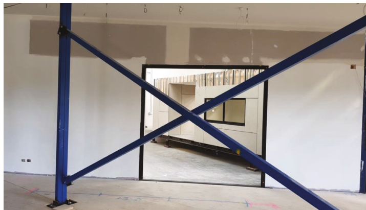
Figure 4. A temporary cross bracing applied between two temporary columns in a prefabricated volumetric module (all to be removed after installation).
