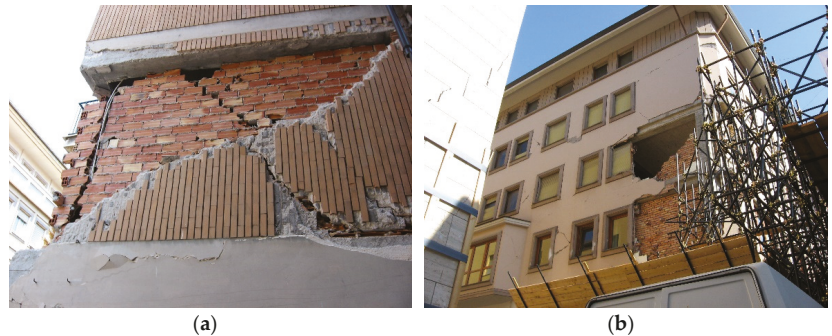
Figure 1. (a). Classic X-shaped infill lesion with intact supporting structure; (b). Typical expulsion of infill masonry wall (Photos taken by the author during the L'Aquila earthquake of 6 April 2009).
