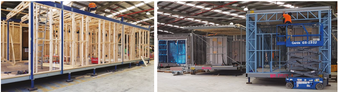
Figure 1. A steel modular unit with softwood wall frames (left) and a steel corner supported modular unit with a cold formed light-gauge steel wall frame (right), showing various materials used in prefabricated construction.
