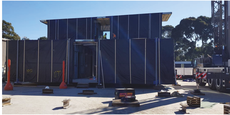
Figure 16. Example of a full-scale prototype carried out within the manufacturing facility of a prefab builder for a double storey-steel modular building to check issues in buildability and installation sequence.
