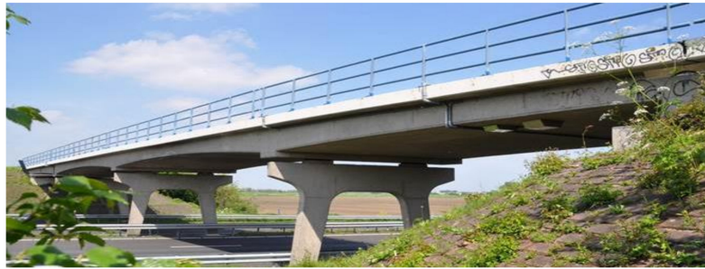
Figure 3. Example of a common four-span plate bridge type in the Netherlands: Bridge Zijlweg of the highway A59 in the province Brabant.
