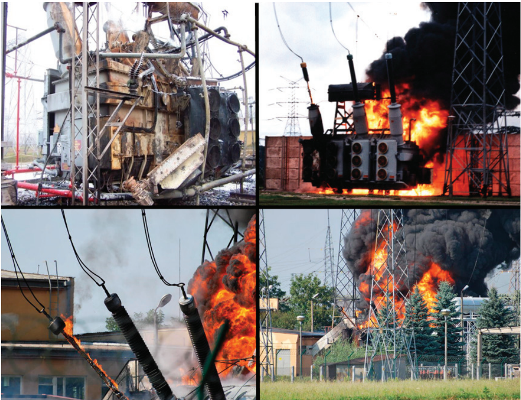
Figure 2. Examples of catastrophic failures of high power transformers initiated by the failure of a bushing.
