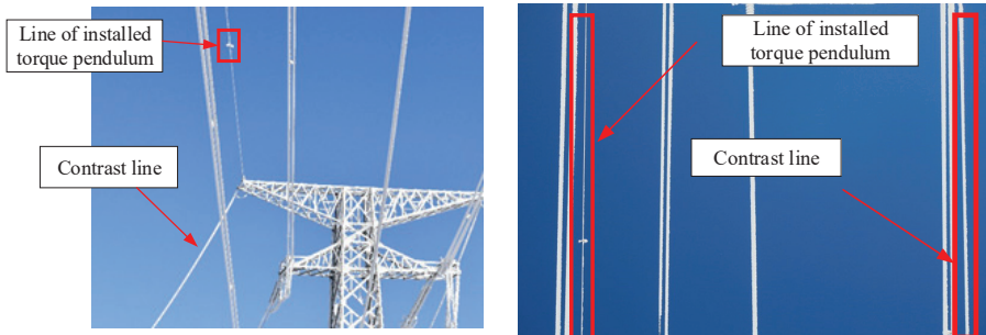
Figure 11. Natural icing contrast of overhead ground line.
