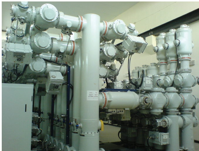
Figure 8. Gas insulated switchgear.
