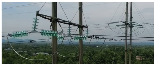
Figure 30. Application of inverted T-shaped insulator strings in transmission lines.
