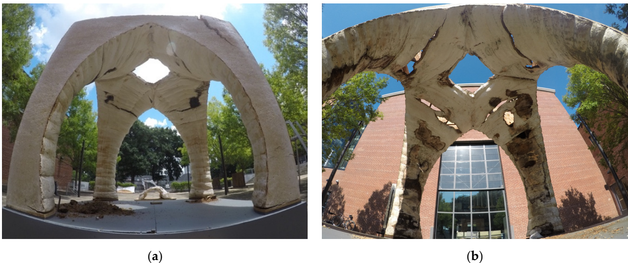
Figure 3. Decay of the Monolito Micelio. (a) Cracking and decay of the structure after three months caused by expansion and contraction of the material matrix against the internal reinforcing structure; (b) cracking, decay, and infestation of the structure after four months. Photos by the author.
