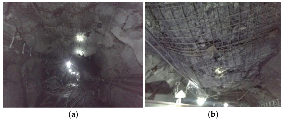
Figure 4. Deformation diagram of partial roadway-surrounding rock. (a) Overall damage diagram (b) Local damage diagram.
