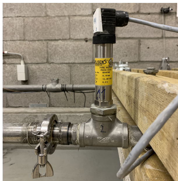
Figure 6. Example of a pressure sensor being screwed in a T-connector as close as possible to the virtual pipe wall.
