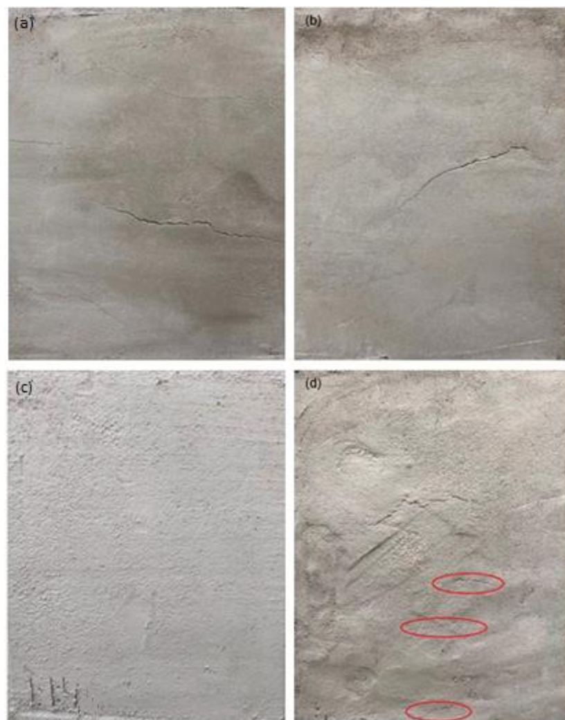
Figure 7. Visualization of cracks presence (red circle). Mixtures: (a) R01, (b) R02, (c) R03, (d) Hydrated Lime.
