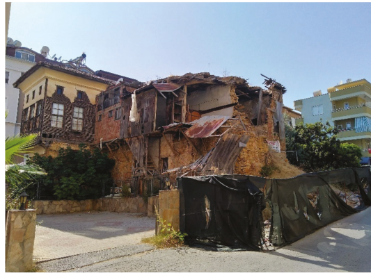
Figure 1. A deteriorated historic building in Turkey.
