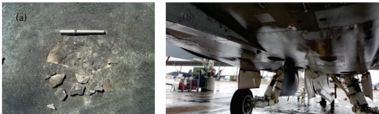
Figure 3. (a) Scaling at the top layer of the military airbase concrete and (b) Underbelly of an F/A-18 with the APU in the centre. Reprinted/adapted with permission from [107]. 2018. Skill.
