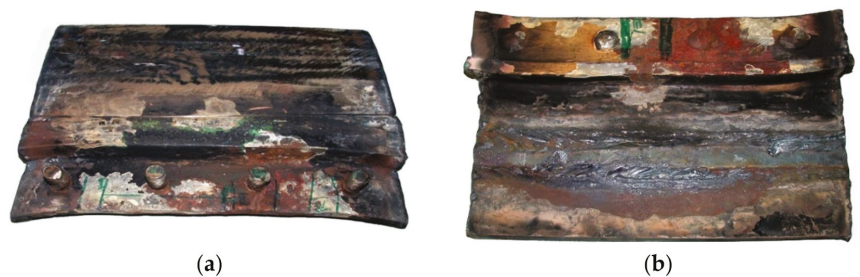
Figure 26. Macroscopic examination results (handy-size bulk carrier 30210 DWT): (a) view of a manhole section from the top of the deck and (b) view of a manhole section from the bottom of the deck.
