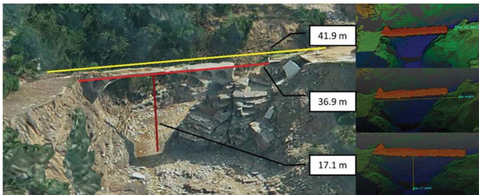
Figure 7. Dam failure site and laser point cloud measurement data.
