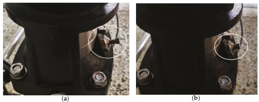
Figure 14. Air binding fault setting: (a) Exhaust screw loose, (b) Exhaust screw tightened.
