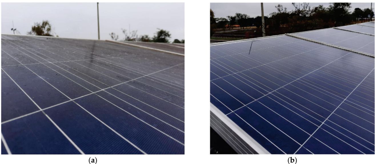
Figure 6. Comparison of the PV modules conditions: (a) before washing; (b) after washing.
