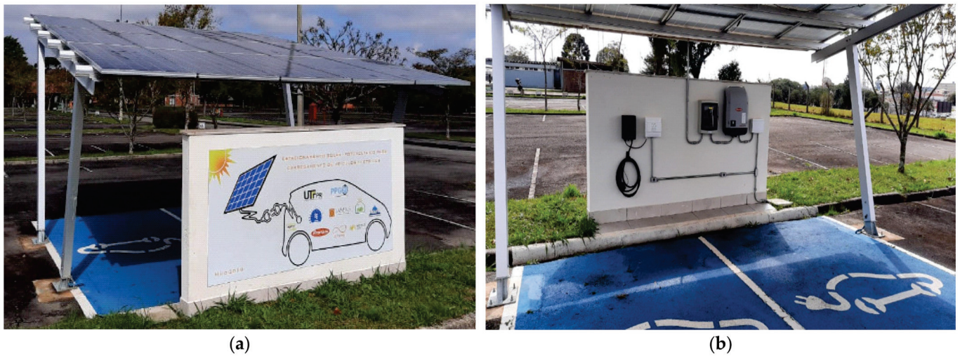
Figure 3. Current carport installations: (a) External; (b) Internal.
