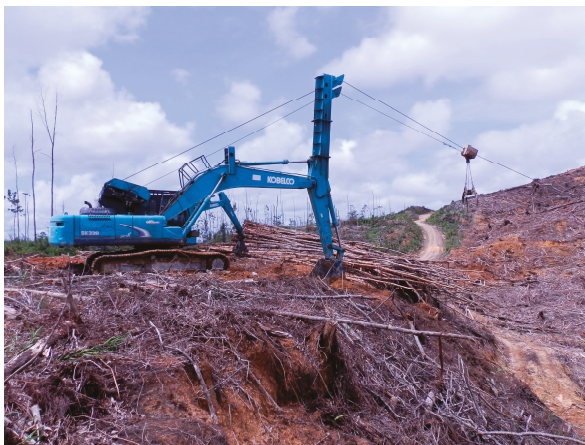
Figure 2. One of the excavator-based un-guyed grapple yarders used in the study (shotgun configuration).
