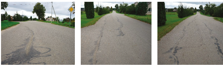
Figure 4. Sealed longitudinal cracks on road No. 2430 in summer 2017.
