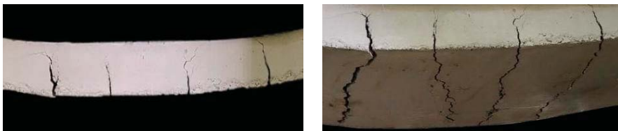
Figure 10. The cracks at the mid-span of the slab: (a) front view; (b) bottom view.
