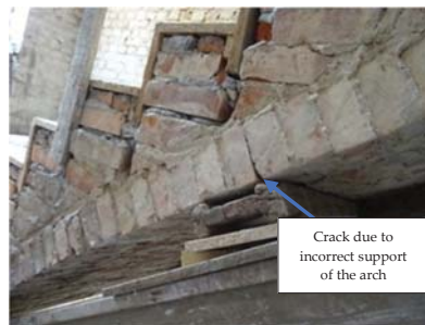
Figure 7. Section of the staircase with visible crack of the arch caused by improper renovation and deterioration of masonry joints.
