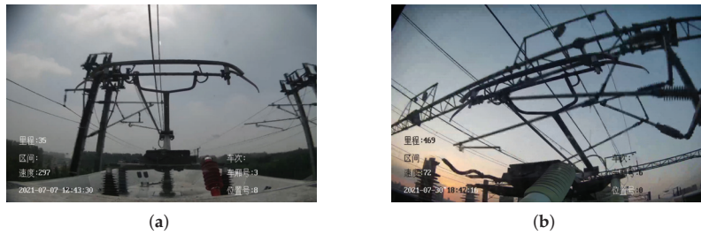
Figure 10. Catenary support device affects pantograph detection. (a) HSR-A. (b) HSR-B.
