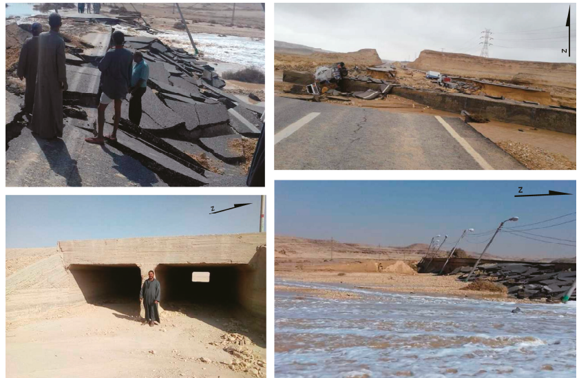
Figure 1. Photographs show the destruction of El Geish highway by the March 2020 flash flood. Source: https://www.youm7.com (Online Newspaper published on 14 March 2020).
