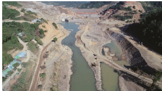
Figure 2. Construction site of the Tha Htay Hydropower Project from downstream view. (Source: survey photo).
