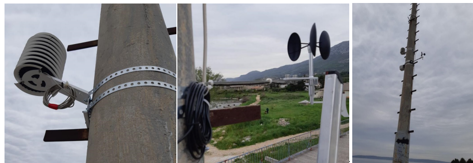
Figure 7. Installation of MeteoHelix and MeteoWind IoT Pro devices.
