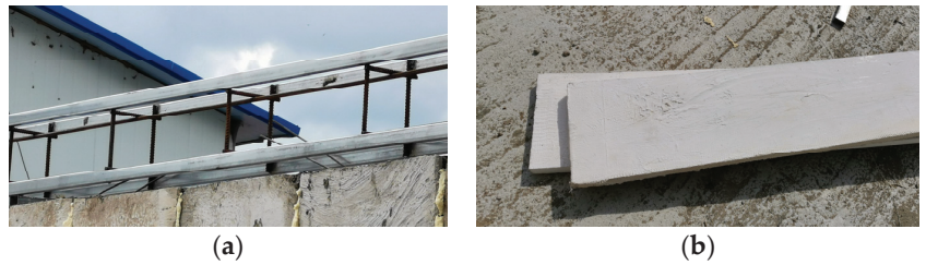
Figure 21. Enhanced reinforcement cage and removable formwork. (a) Improved reinforcement cage for beams; (b) improved XPS formwork for easy removal.
