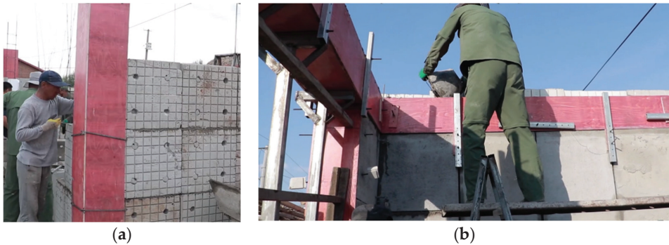
Figure 5. On-site construction of beams and columns. (a) Pouring of columns. (b) Pouring of beams.
