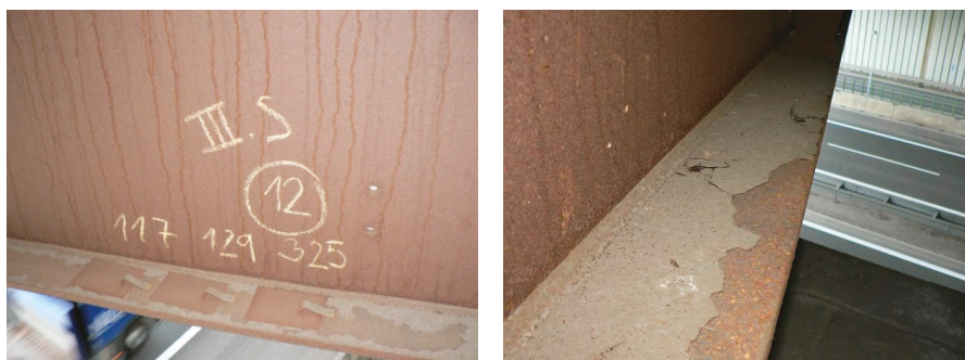
Figure 8. Bridge No. 1—unfavorable development of corrosion products on the internal upper surface of the bottom flange (surface P6).
