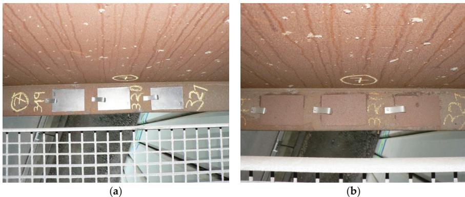
Figure 5. Corrosion samples on the upper surface of the bottom flange at the time of installation (a) and after 1 year of the exposure (b).
