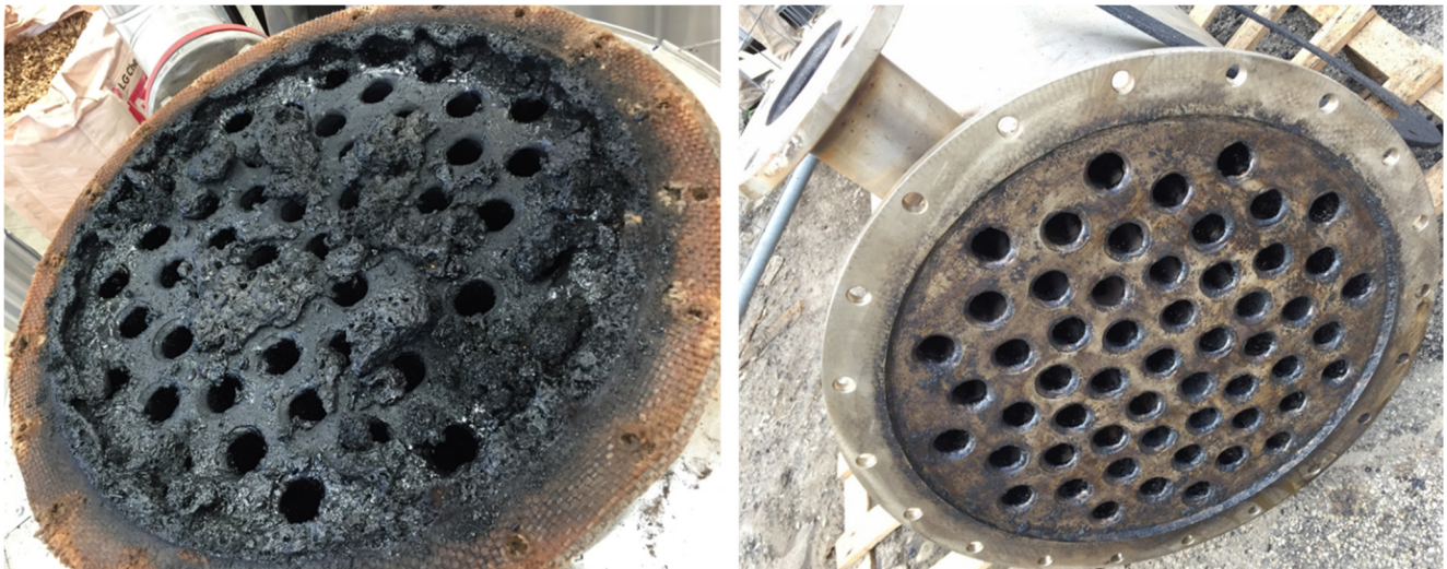
Figure 11. Upper tube plate before (left) and after (right) mechanical cleaning.
