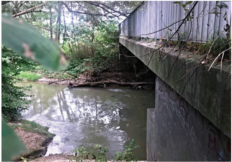
Figure 9. Current state of preservation of the Dlubnia inundation area, 2021.
