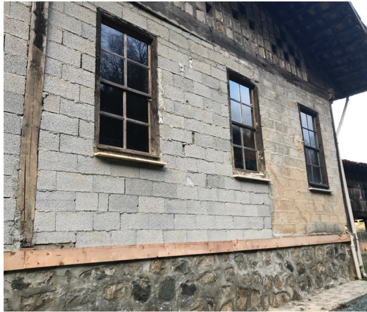
Figure 7. Site visit of a house in Çaglayan village in Fındıklı on 12th January in 2019. Maladaptation example of rebuilding the eradicated rear façade with briquette wall after the landslide in 2018. Source: Photograph by the first author.
