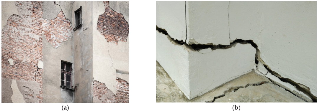
Figure 1. Examples of damage in (a) masonry or (b) concrete structures (figures reproduced with permission from Unsplash).
