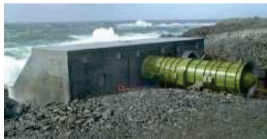
Figure 7. LIMPET OWC plant (Sun et al. 2018 [24]).
