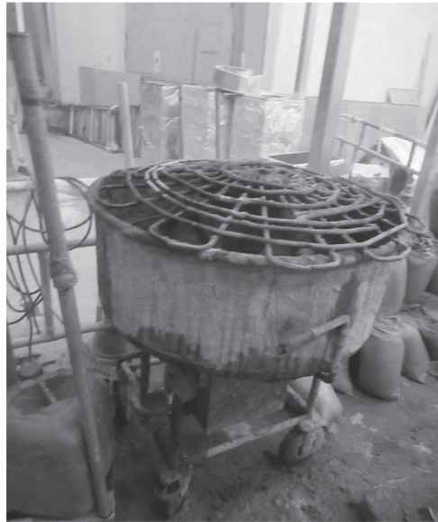
Figure 7. Wet cement sand mixing for building a brick wall at a renovation site.
