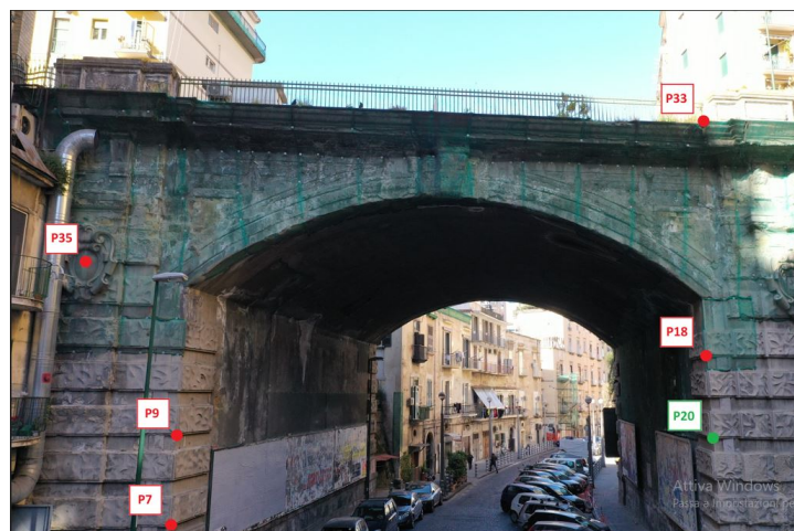
Figure 5. View of the south facade with markers locations. GCPs are represented in red while CP is represented in green.
