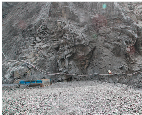
Figure 1. Slope rock mass of the left bank near the dam site of the Lianghekou Hydropower Station.
