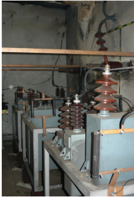
Figure 11. Damaged capacitor battery used to compensate for the reactive power of the arc furnace.
