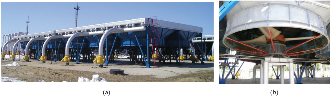
Figure 1. Gas cooling plant (a) and VASO-16-14-24 electric motor with a fan on shaft (b).
