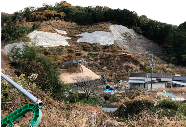
Figure 2. Ongoing road restorations and slope protection constructions in the Hiraenoki Community (obtained by Yoshio Harada [the first author] on 12 December 2019).
