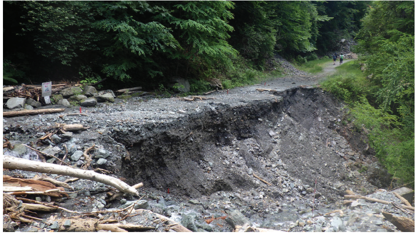
Figure 1. Image of forest road failure. A culvert at a stream crossing was destroyed by heavy rain, and the road body was eroded by stream water, making it inaccessible to vehicles.
