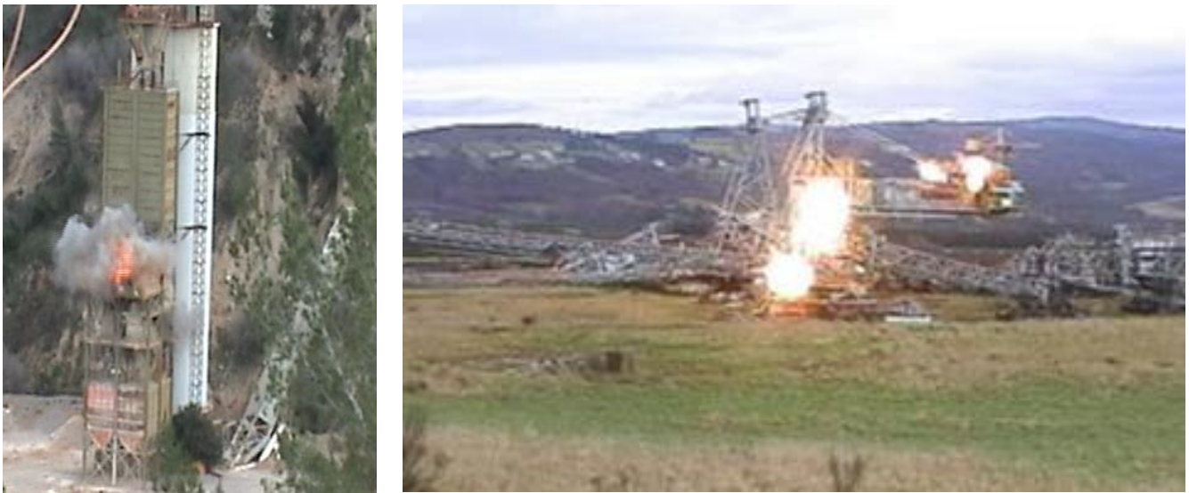
Figure 5. Demolition of metallic structures with shaped charges ((left) metallic silo; (right) large mining stacker).
