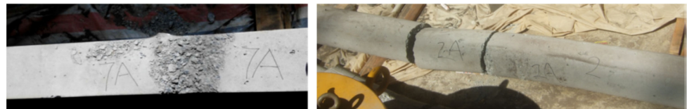
Figure 10. Columns after blast test [24]. Copyright permission obtained from authors.
