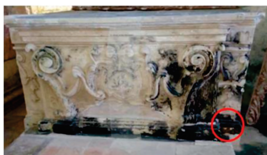
Figure 2. Black crusts on the altar of St. Joseph in the San Pietro Barisano church.
