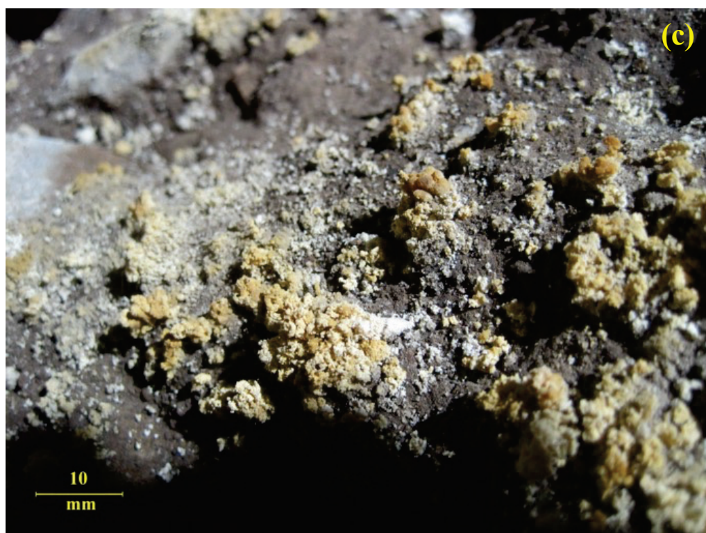
Figure 2. Photos of the degradation (a) of the floor and (b) of the wall and optical microscope image (c) on the surface of the black and white mosaic pavement (10× and 40× magnification, respectively; width focusing 25 mm, 2 mm increments; 6 V/20 W halogen light). The sample of the degradation product of the black and white pavement mosaic of domus B was analyzed under an optical microscope in transmittance and reflectance).
