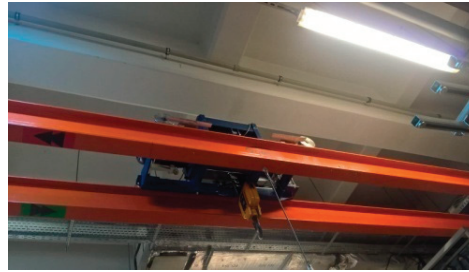
Figure 2. The tested double-girder overhead traveling crane with a trolley and a hoist.
