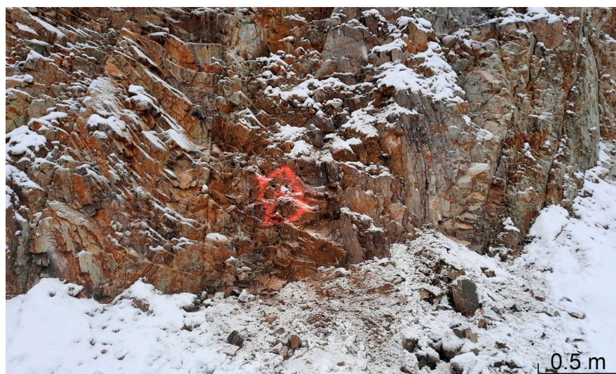
Figure 2. Weathered, strongly jointed granulate, corresponding to (2).
