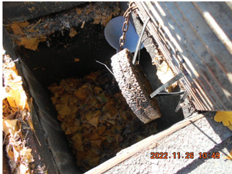
Figure 14. Hanging-type placement of the porous concrete at the same inlet as the one shown in Figure 1. The grating is open. Closing the grating results in the porous concrete board assuming a horizontal orientation.
