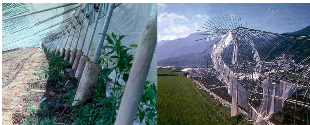
Figure 1. Case of foundation damage of single-span plastic greenhouse [27].
