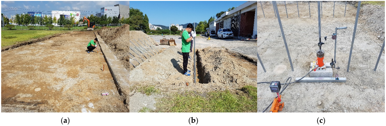
Figure 4. Field test procedure of site A: (a) ground grading work; (b) embedded depth leveling; (c) uplift testing of continuous foundations.
