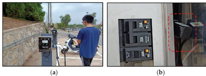
Figure 11. (a) Field picture with charging piles, (b) power distribution box with an IoT clamp-meter marked in red.
