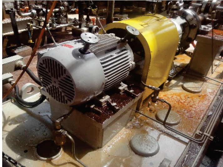
Figure 3. Industrial electric motor driving a wastewater pump.
