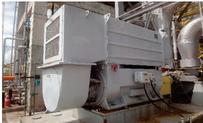
Figure 4. Industrial electric motor driving the principal centrifugal pump.
