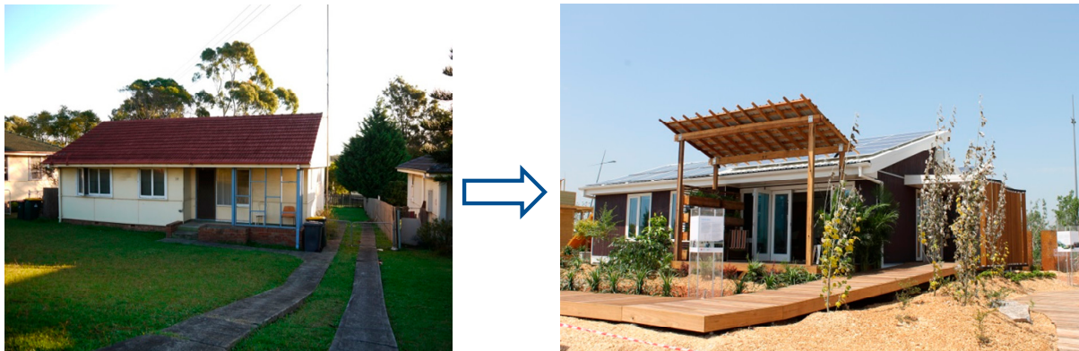
Figure 9. Illustration of deep retrofit of a typical Australian timber framed fibro house.
